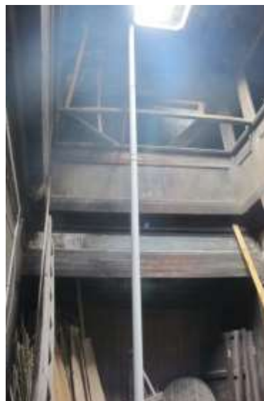
Figure 2-5 The damaged roof of a house near Wu's Ancestral Hall (No. 29, Dongbianjing) is supported by a wooden stick.
