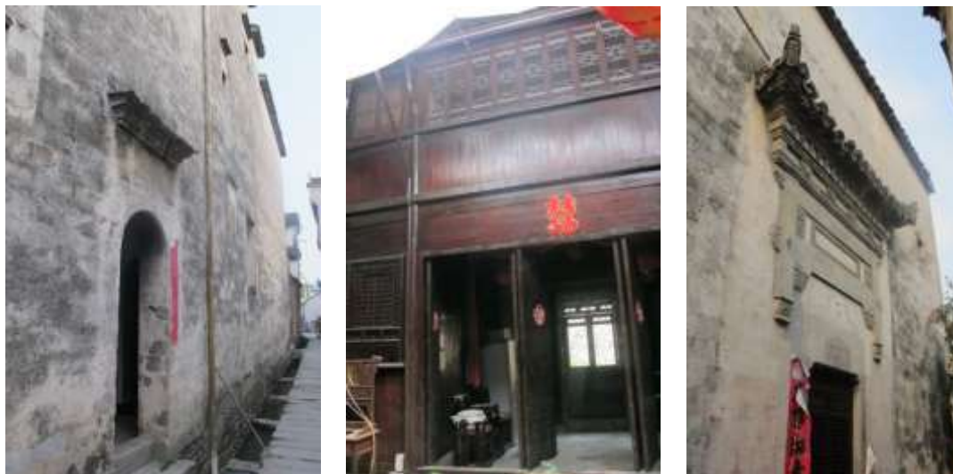
Figure 2-16 Left: Side door of S15 on the roadside; Middle and right: Closed front door of S15
